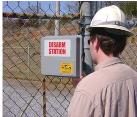
A disarming system allows entry for utility personnel and approved contractors, but keeps copper thieves out.
