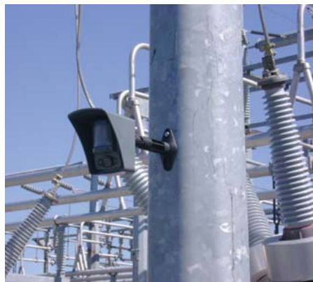
A wireless video camera system keeps constant watch over a substation.
